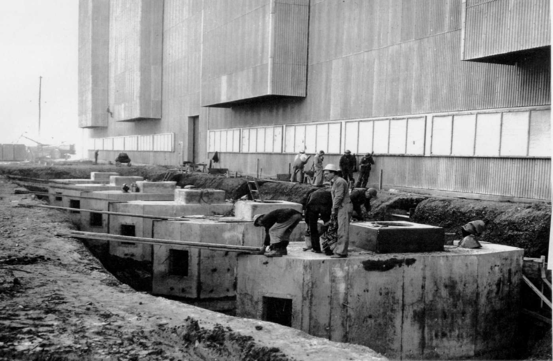
U. S. A. E. C. PADUCAH AREA OUTSIDE ELECTRICAL DISTRIBUTION SYSTEM N. OF PROCESS BLDG. C-337 55% COMPLETE F. H. MCGRAW & CO., CONTRACTOR AT-(15-1)-2 2-10-54
